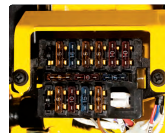
An Accessible, Compact Fuse Box for Easy Inspection
