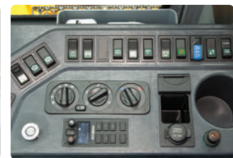
Centralized Instrument switch Panel
